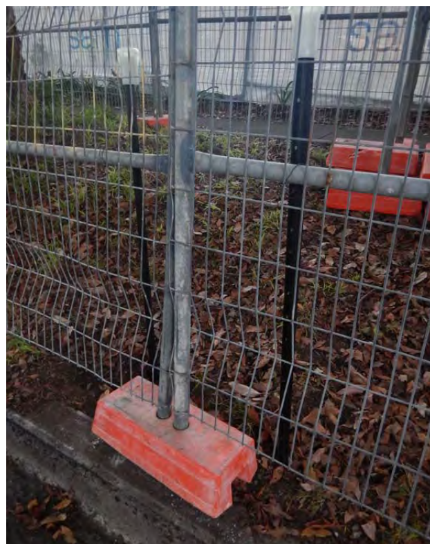
Figure 92- Where ground is uneven or the site is subject to strong winds the fencing may be held securely by wiring to strategically placed star pickets driven into the ground. (Photo: Arterra)
