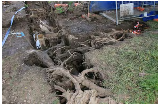
Figure 96- Non-destructive excavation methods can allow services to be installed across verges without the need to sever important and structural tree roots. (Photo: Arterra)
