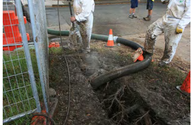
Figure 95- Hand excavation or other non-destructive methods such as water jetting and vacuum extraction to excavate around tree roots. (Photo: Arterra)
